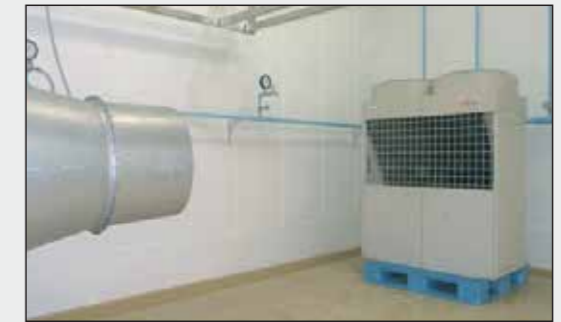
Shower Test Room
